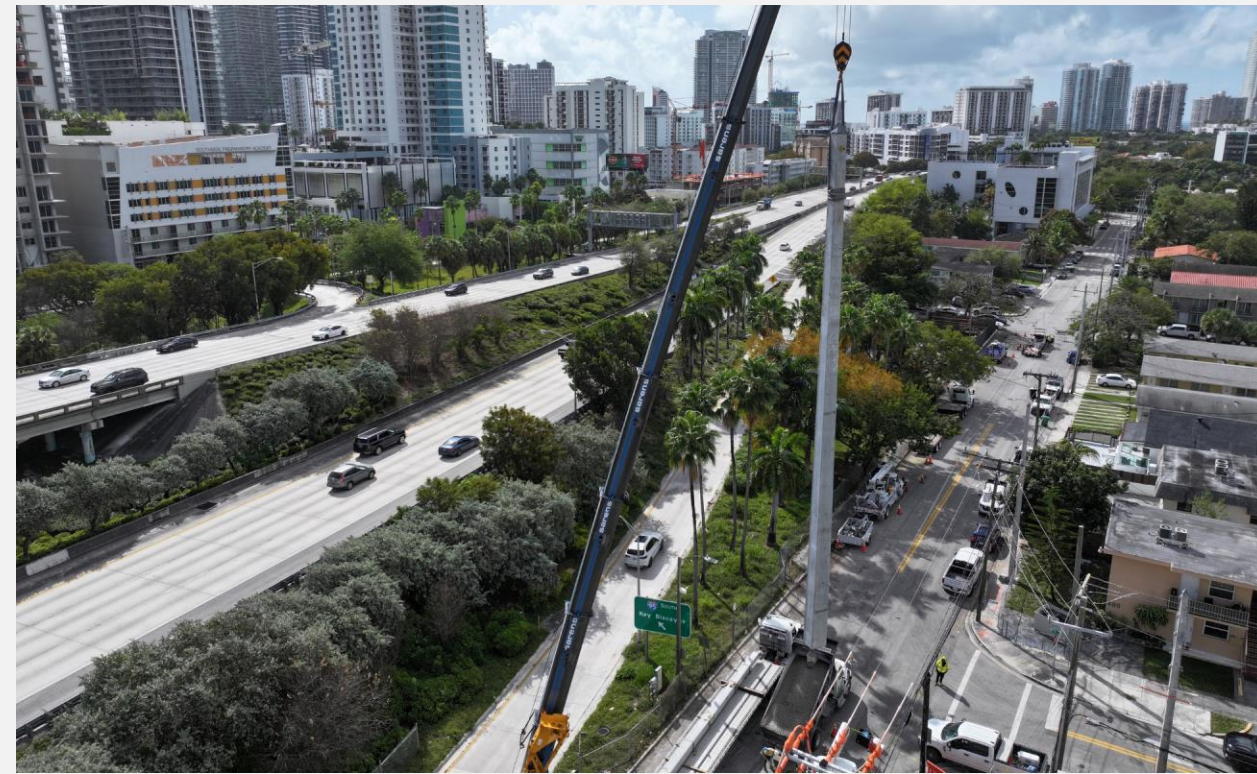
Year-round grid hardening to prepare for hurricanes and severe weather
